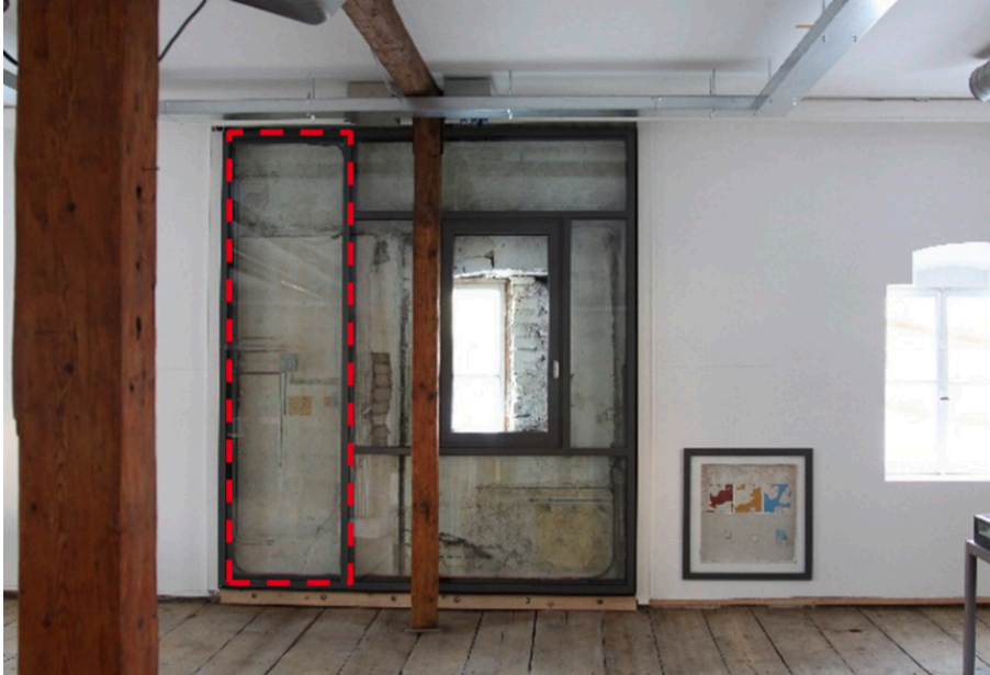
Figure 1. Transparent internal wall insulation on the west-side in the upper floor of the Alte Schöfferei. The left part of the transparent internal wall insulation (dashed rectangle) is examined and evaluated.
