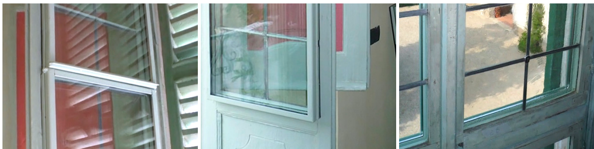
Figure 2. Example of installation of a secondary external glazing in Villa Piazzi in Nerviano (MI) by the restorer Ercole Livio Rini. (a, b) View of the external side. (c) Inside view of the closed window.
